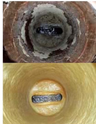
CIPP manhole rehabilitation before (top) and after (bottom). Pictures courtesy of Poly-Triplex.
