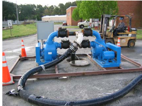
A typical large-capacity bypass pumping system working from an existing manhole. Picture courtesy of Hampton Roads Sanitation District, Virginia, USA.
