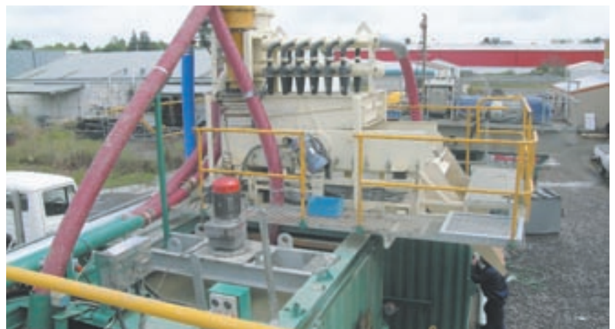
■ Slurry separation tank.
