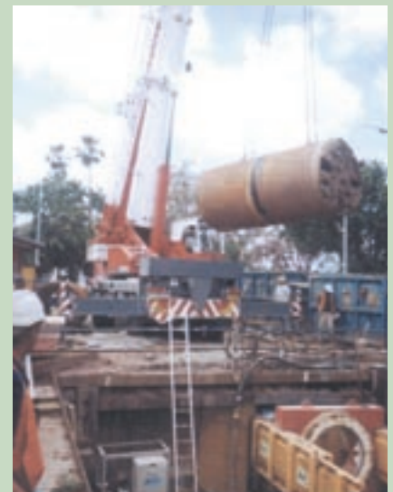
■ AVM 120c Tunnelling machine being placed on jacking rails at launch shaft.
