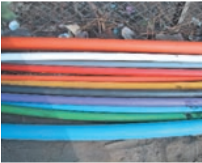
■ 12 x 40mm ducts
