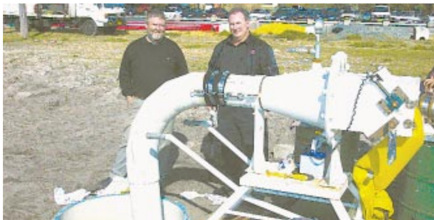
■ ShieldLiner Chief Executive John Hassen (left) and Premium Corporation Director Trevor Gosatti at the field trial of ShieldLiner's pipe repair system.
